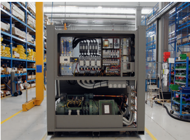
Uniflair's 600 kW water cooler features a silent air condensing system and a redundant power supply. The automation solution protects the unit against over-voltage and phase distortion.
